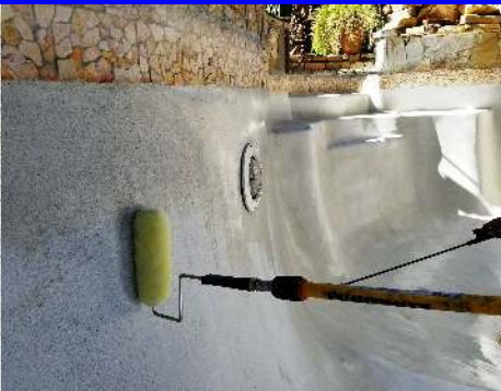
Now the sprayed section is being back rolled with a dry roller.
